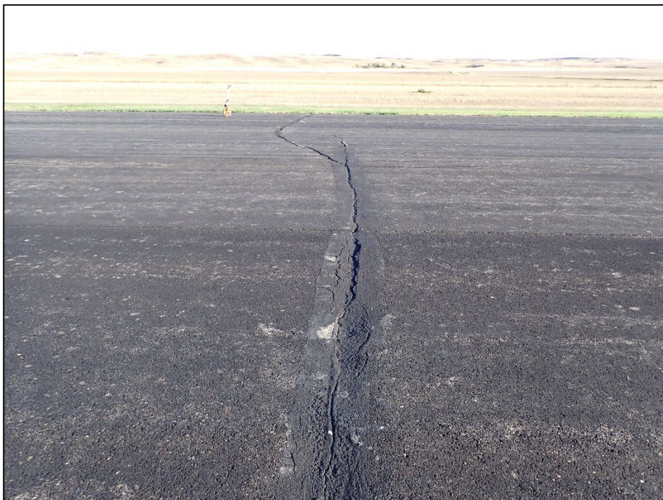
RW08-02-02: L&T Cracking
