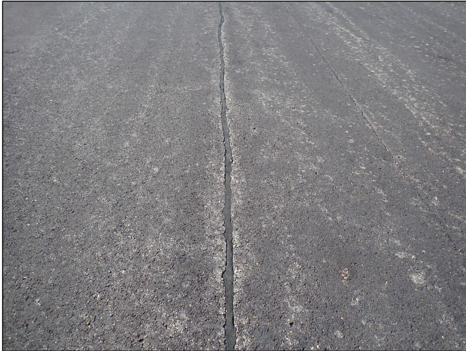
AP-01-02: L&T Cracking
