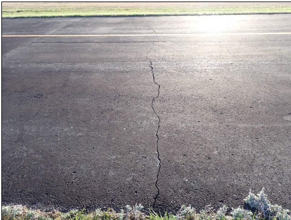
TW-02-01: L&T Cracking
